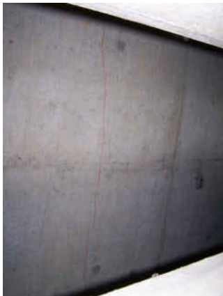
2131513_0_2009H_K-WAND WL-V GERISSEN
