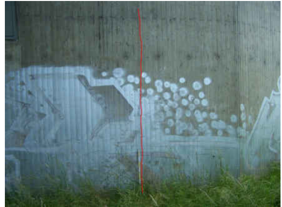
2131513_0_2009H_WL-V LINKS GERISSEN
