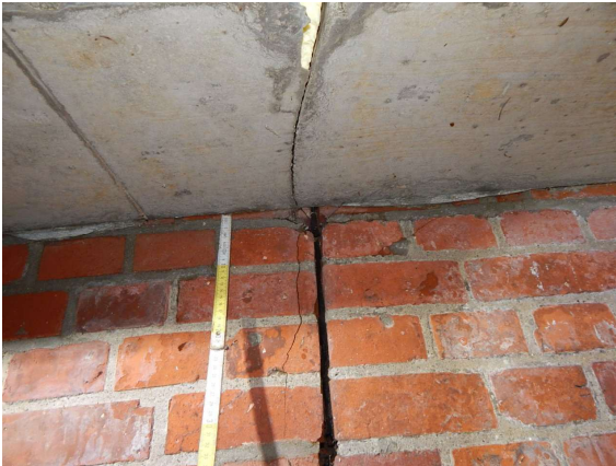
ASL_030_0_2025H_L-STW H-FUGE OBEN FLANKE GERISSEN
