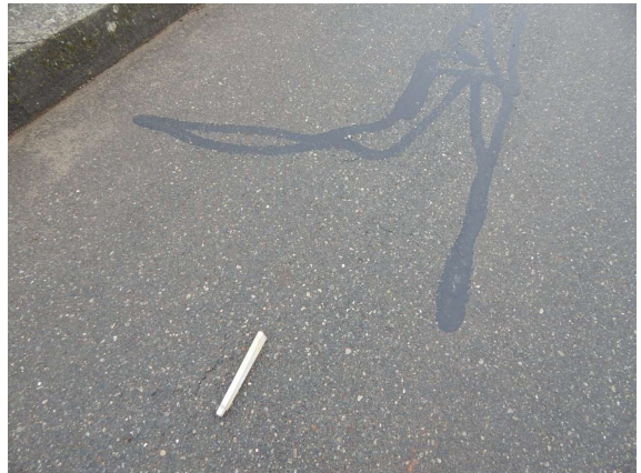
ASL_027_0_2025E_BELAG MITTIG LINKS RISSE
