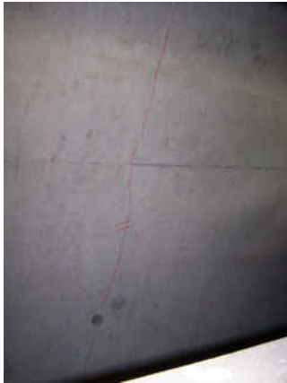
2131513_0_2009H_K-WAND WL-H GERISSEN
