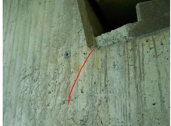
2131506_0_2009H_WL-H LINKS GERISSEN
