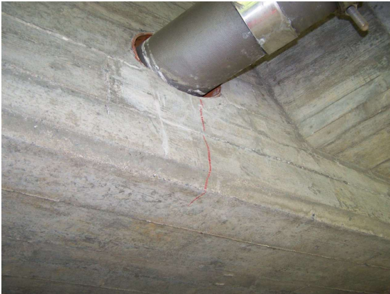
2131506_0_2009H_EQT-V HINTEN LINKS GERISSEN
