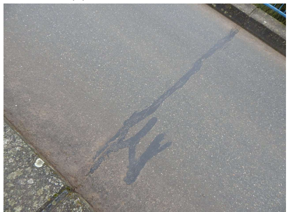
ASL_027_0_2025E_BELAG VORNE QUERRISS
