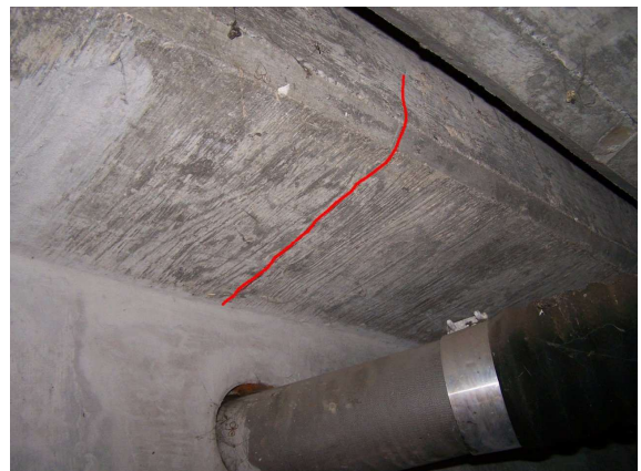
2131506_0_2009H_KONSOLE FUK EQT-V GERISSEN
