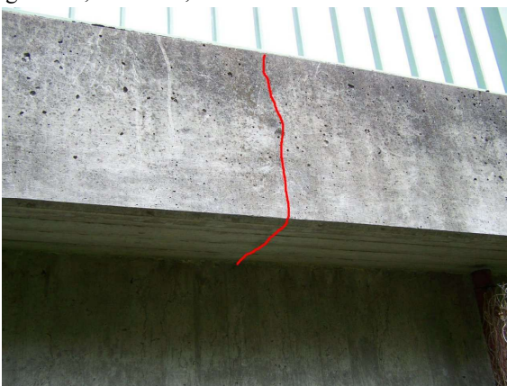
2131506_0_2009H_GESIMS H-R-FL WL-2 GERISSEN
