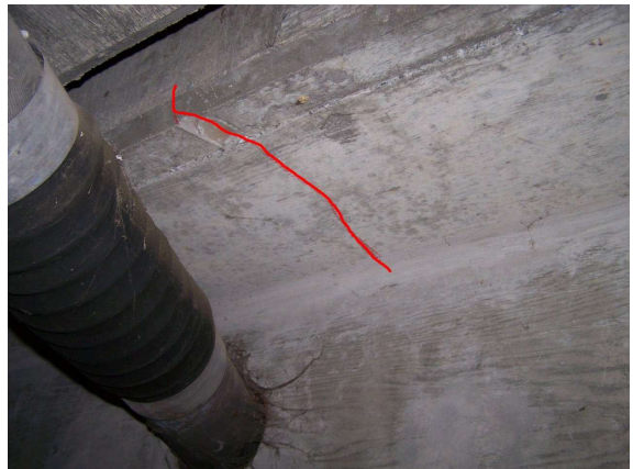
2131506_0_2009H_KONSOLE K-WAND-V GERISSEN
