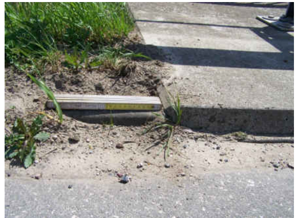
2131513_0_2009H_H-R-BORDSTEIN ZU TIEF
