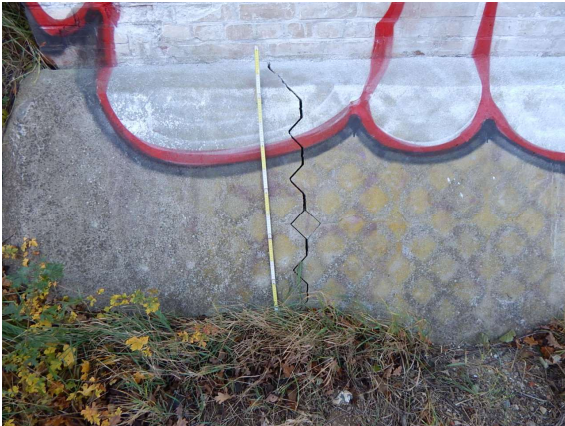
ASL_030_0_2025H_WL-V RECHTS-GERISSENE BERME
