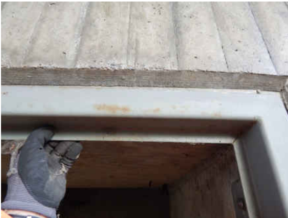
2131513_0_2019H_TÜR WL-H OBEN ANGEROSTET
