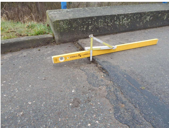
ASL_027_0_2025E_BELAG VORNE LINKS ABSACKUNGEN
