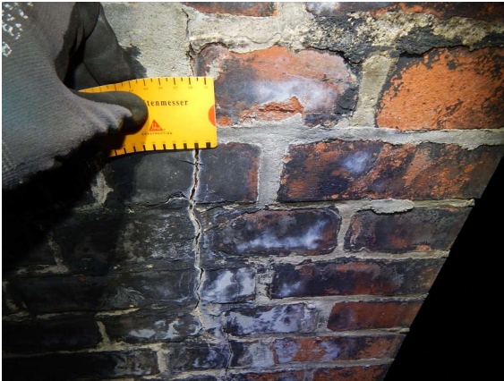
ASL_030_0_2017H_GEWÖLBE LINKS MITTIG-STIRNRINGABRISS
