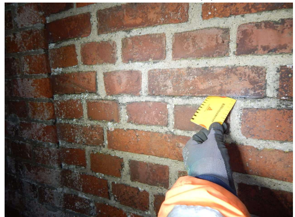
ASL_030_0_2017H_R-STW VORN FUGEN GERISSEN
