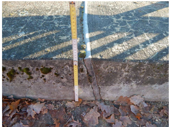
ASL_032_0_2025H_L-KAPPE VORNE FUGE SCHIEF
