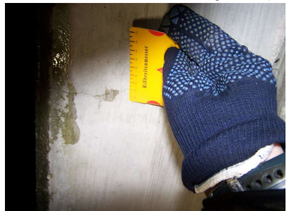
ASL_032_0_2013H_L-GESIMS MITTIG QUERRISSE
