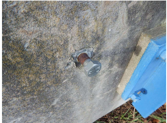
ASL_032_0_2022E_L-FL WL-V BOLZEN ANGEROSTET
