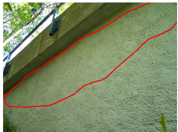
ASL_032_0_2013H_R-FL WL-V OBEN HOHLSTELLEN
