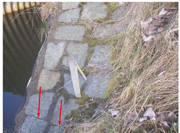
ASL_029_0_2009H_R-STIRNRING FUG BRÜCHIG
